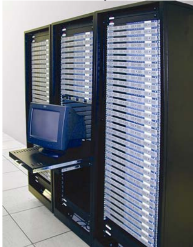
Rice University Datacenter
