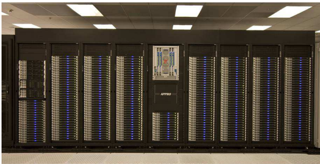
Figure 2: Graph Cluster on datacenter floor at LLNL
